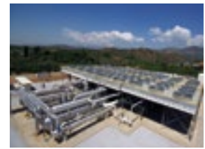
Turkey Geothermal power Dora II
