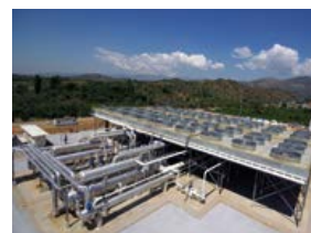
Turkey Geothermal power Dora II
