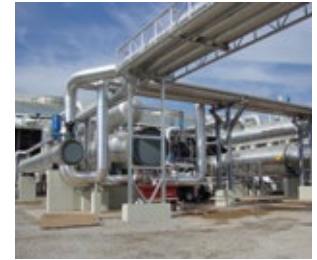
Turkey Geothermal power Dora II
